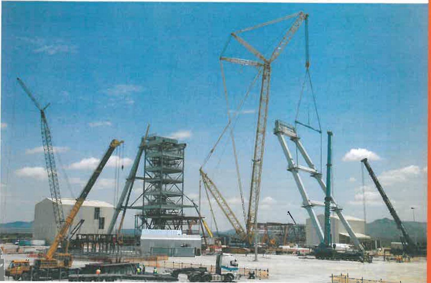
The Styldrift site showing headgear erection using a 1 000-t lattice boom crane. Shaft Sinkers is sinking the main and vent shafts for Styldrift (photo: TWP).
