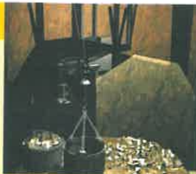
Shaft Sinkers has developed a technique which utilises the lashing unit to move the kibbles at shaft bottom.
