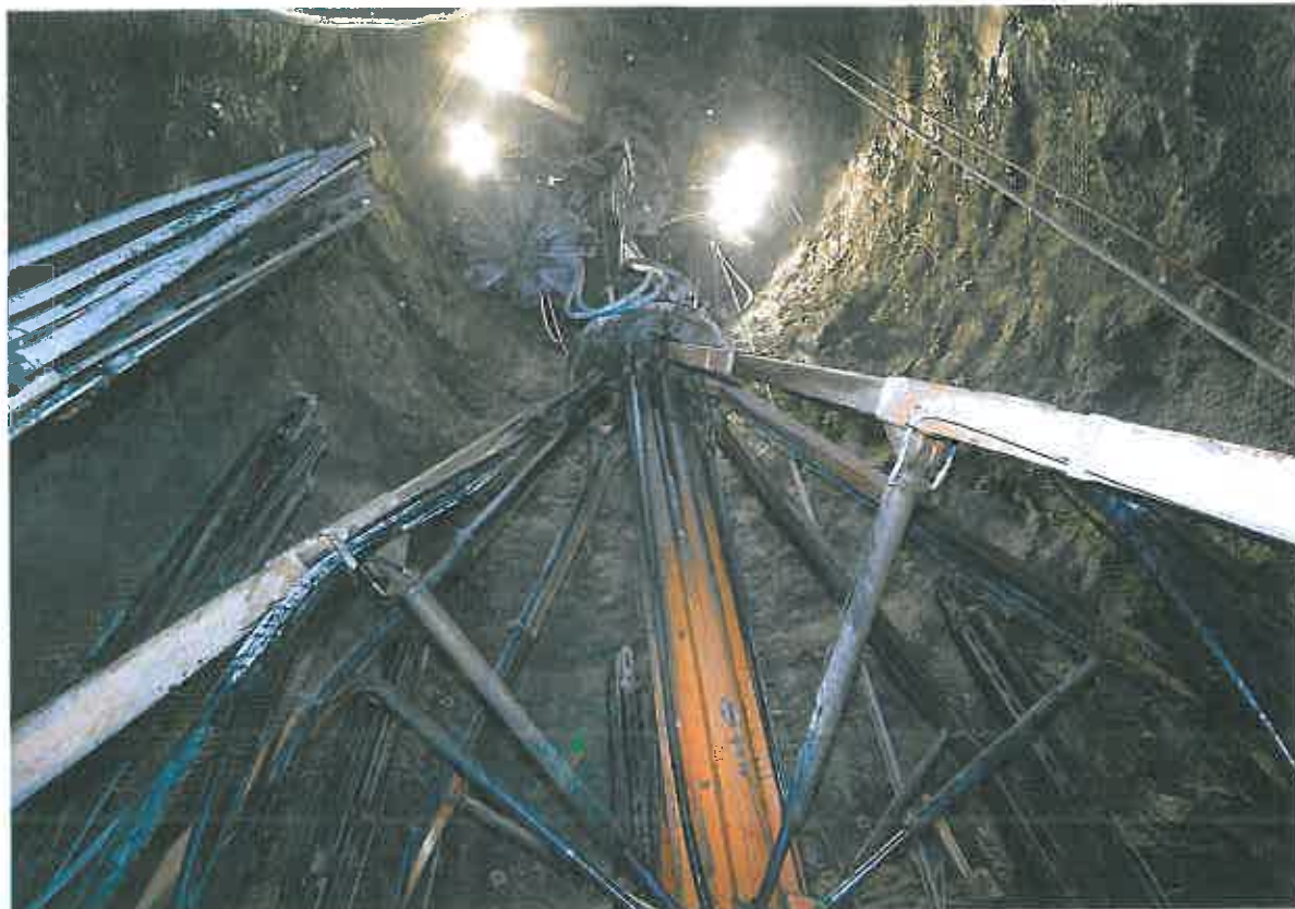
Shaft Sinkers is sinking three deep shafts at Impala's No 17 Shaft complex. Seen here is the vent shaft, which will go to a depth of just over 1 700 m (photo: Alf Yssel).
